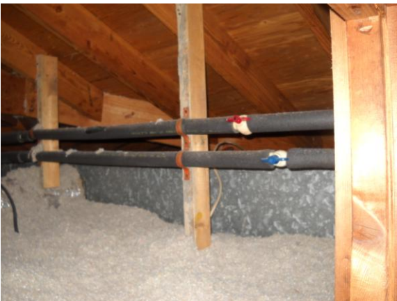
Shut-off valves in attic above laundry room
