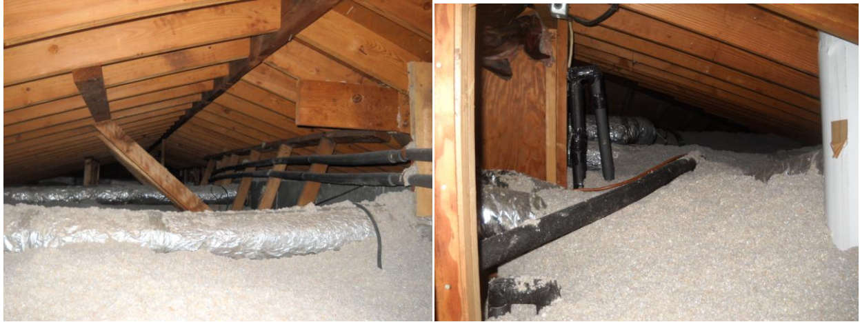
R-19 to R-30 loose-fill wood fiber insulation in attic - Properly insulated CPVC re-pipe through attic
